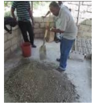
Build Change engineer Emmanuel Architecture for to properly mix concrete to block makers
